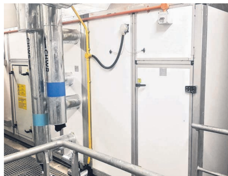
One of the two air handling units (AHUs) on each floor of Guoco Tower, which prevents cross-contamination between floors. When both AHUs operate at full capacity, the air in the office space is fully circulated five times every hour. PHOTO: GUOCCOLAND
